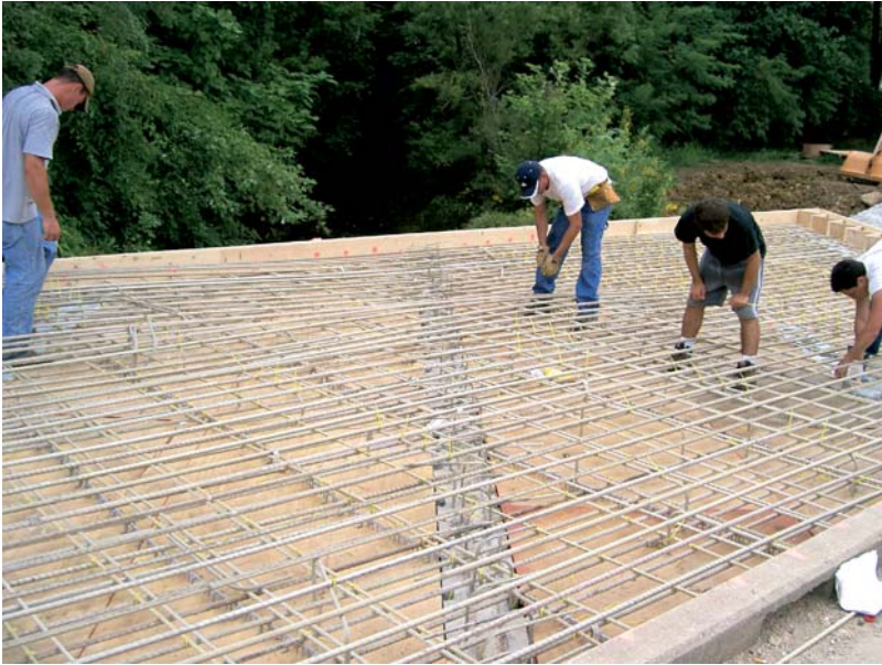
Fig. 2 Setting a FRP network for casting a construction concrete in the repair of a bridge (Courtesy of D. Gremmel, Hughes Brothers)
